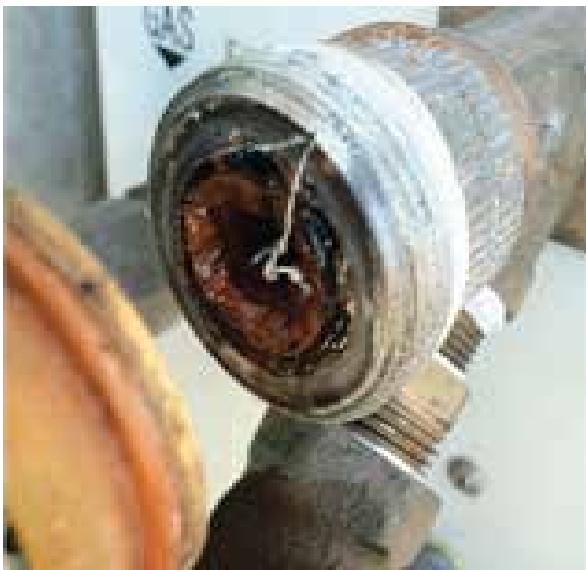
Fig. 2 Corrosion within a plumbing pipe where two dissimilar metals have been welded together
